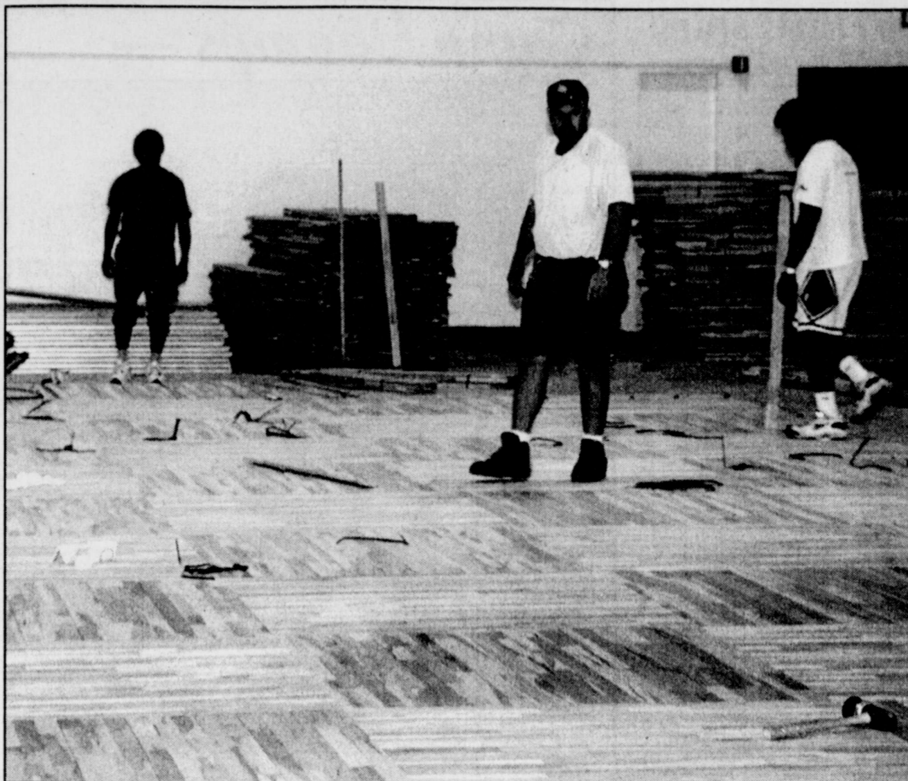
NEW FLOORING is being installed at the Winters gymnasium, under the supervision of maintenance supervisor Dale Montgomery, second from right. The large Boston parquet 50" squares are laid in opposite directions on the playing floor with a standard wood pattern around the playing area. Montgomery said the work should be completed by the third week in September on the new floor which was needed to replace the old flooring damaged by flooding.
