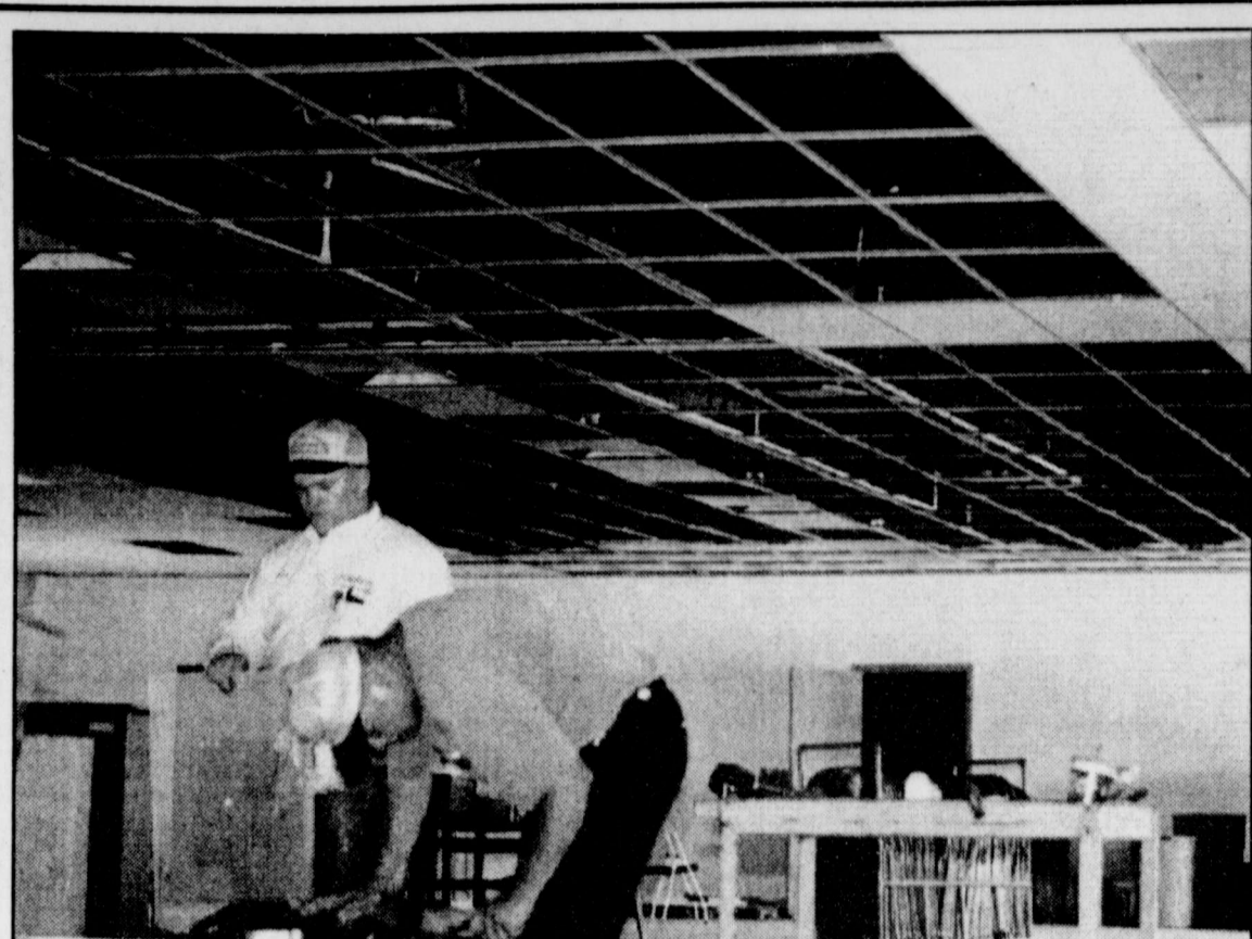
KENDRICK HEATING & AIR CONDITIONING employees James Galvan and Benny Owens have been busy installing the new systems in the renovated Community Center which will have central heat and air conditioning. Work is expected to be completed next week. For new rental rates, call City Hall at 754-4424.
