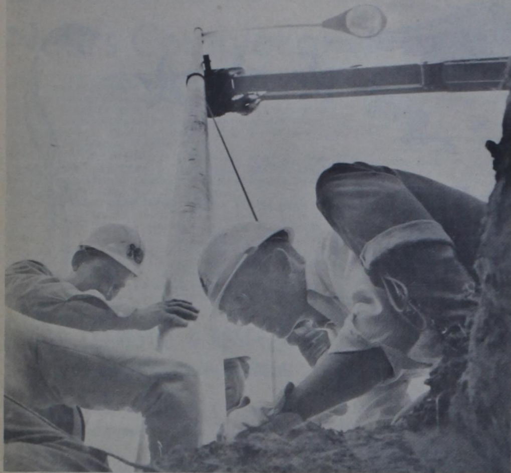
MOLE'S EYE VIEW of street-light construction on the courthouse square shows L. D. Atwood, John P. Smith and Ted Underhill of Southwestern Public Service Co. working at the base of a new 54,000-lumen mercury vapor light. Visitors to the court-
