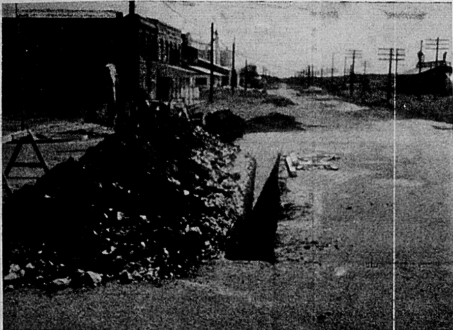
NEW WATER MAINS — Photo shows water mains being laid for the City of Baird. The view is looking East of First Street. Progress to this point is directly in front of the T&P Depot and about the middle of Market Street. (Staff Photo)
