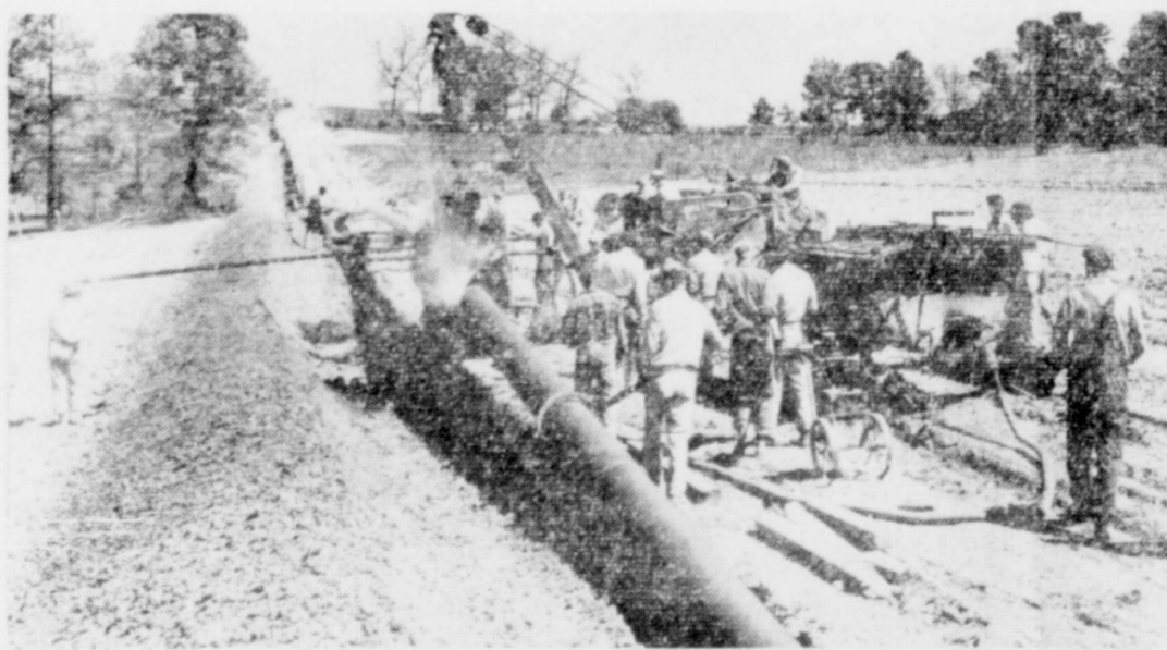
Immediately following the end of war, Lone Star launched an eight-million-dollar improvement program. This program is proceeding just as rapidly as availability of steel pipe, regulators, compressor engines, etc., will permit. Above is scene along right-of-way during construction early last summer of 80-mile high pressure line from great Carthage gas field in East Texas.
