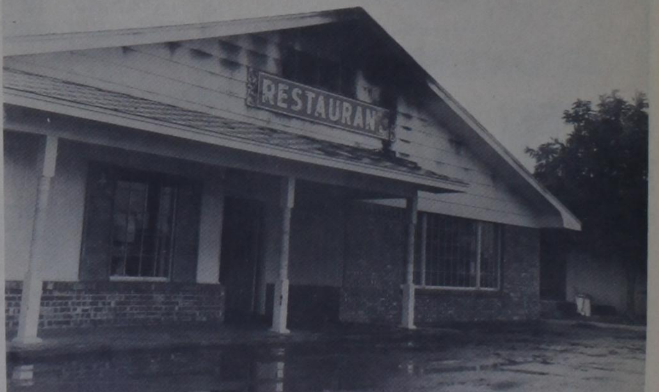
A DEFECTIVE SIGN started the blaze that damaged roof, furniture and carpeting in the Colonial Inn Restaurant and manager's
