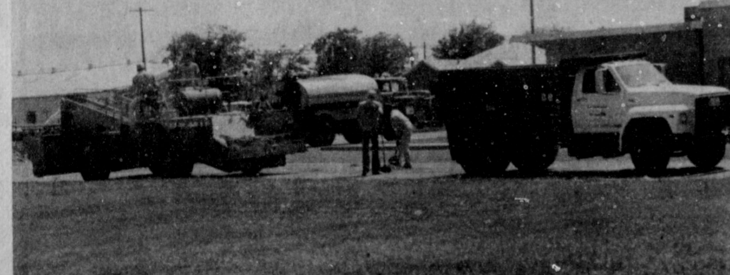
A CREW OF MEN with HI Plains Pavers of Plainview put finishing touches on Second Street east of the City Hall Monday to complete the 23-block project of repairs and resurfacing of town streets.
