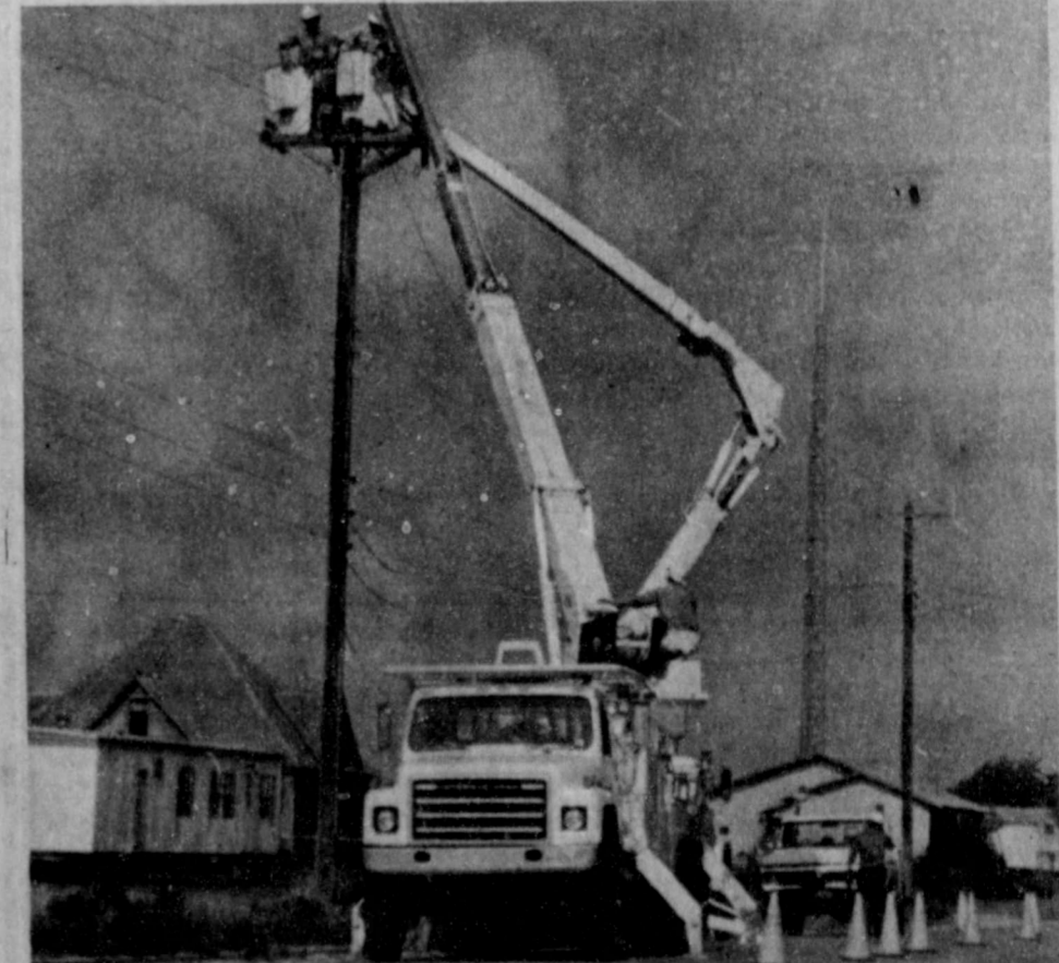
SOUTHWESTERN PUBLIC SERVICE crews worked Monday morning to replace a broken utility pole on East Locust Street. The SWPS reported they had not had to replace any poles because of damage from the recent weather. The only damage caused by weather had been to transformers, cutouts, and insulators.
