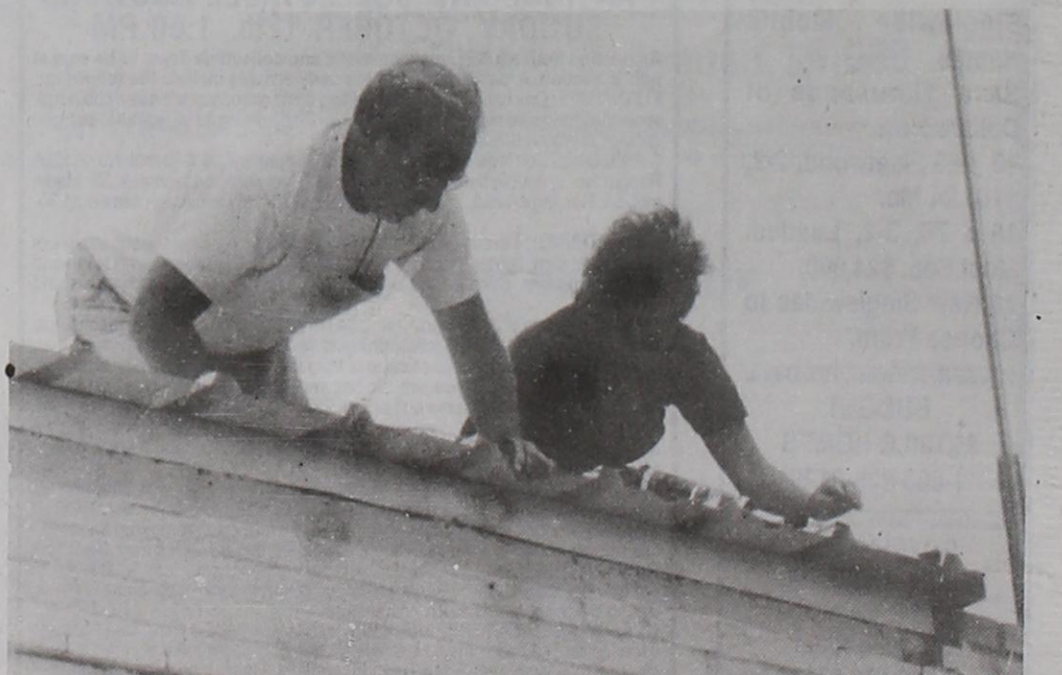
Star Attraction .... Bun Barry (left) and Karen Riddle (right) are shown on top of a building in downtown Baird installing the new Christmas lights. Barry and Riddle are just a couple of the volunteers seen around town on Tuesdays installing the new decorations.
