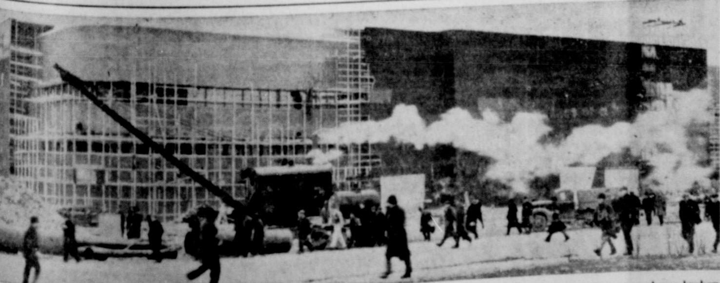
Workers have begun tearing down the huge fiberboard canopy sheltered the $21,000,000 Ford airplane engine plant at Dearborn, Mich., during winter construction. This view shows the front of the plant. The entire building will be completed early in April—little more than six months from the time ground was broken. Ordinarily such a project would require 12 to 14 months, but the shelter built over the structure enabled crews to work around the clock through the dead of winter.
