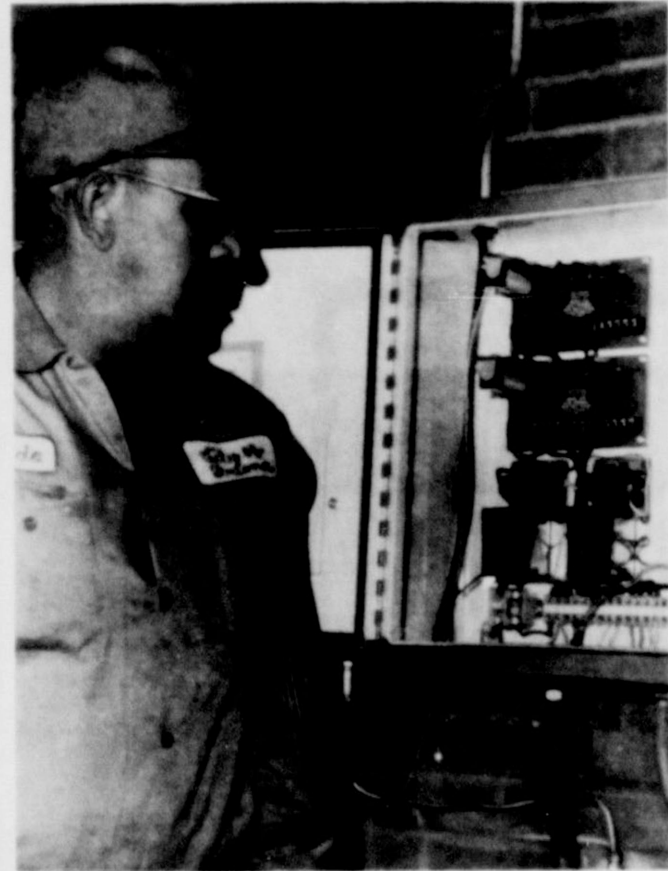
CONTROL BOX. . . . City water superintendent Clyde Fields inspects the new computerized control panel located at the East Plant in the city's water system.
