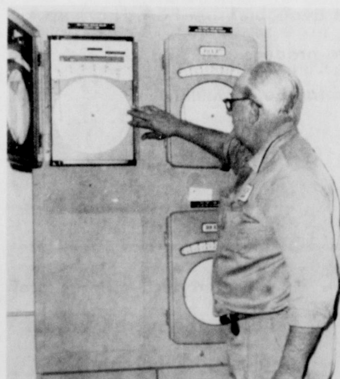
SYSTEM BRAINS. . . . All of the information collected by the city's new water control system is fed into this central control panel, which keeps a record of water pressure throughout the system. Clyde Fields checks a reading.
