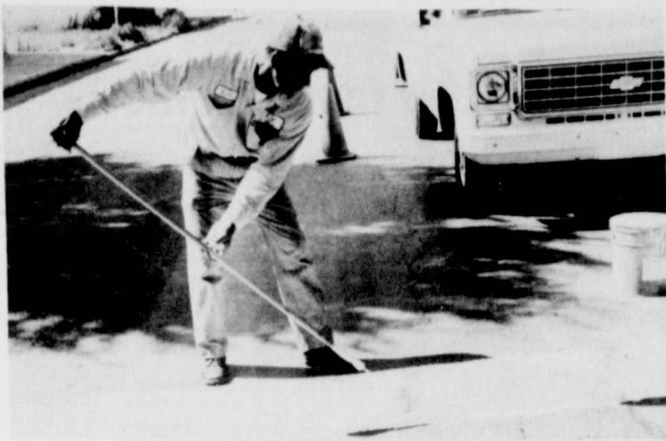
PAINTS CROSSWALKS....A City of Friona employee is shown painting the crosswalks at one of the school crossings in preparation for the first
