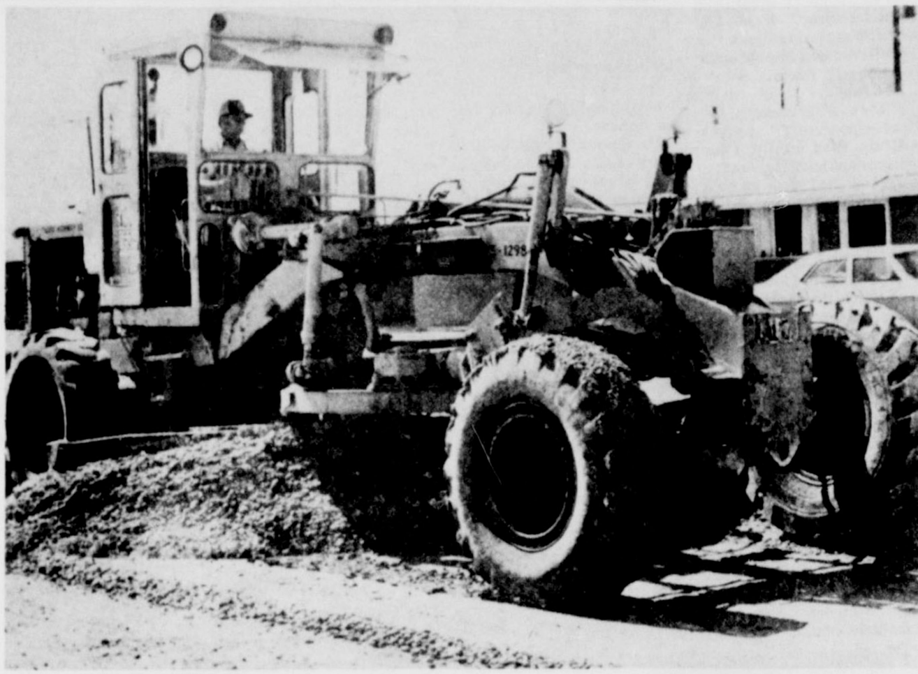
FIXING IT UP ...Road work is in full swing on the west end of Fifth Street. In the above photo a maintainer is shown spreading the calche along the road which is being
