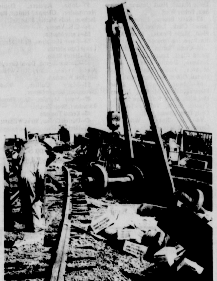
JIG-SAW PUZZLE... Just a portion of the mess that ensued last Saturday after 21 cars of a Santa Fe freight train were derailed just southeast of the Friona City limits. Santa Fe crews worked throughout the day to clear the tracks and had traffic restored by 5:15 p.m. that afternoon. The derailment scattered wrecked boxcars and their contents along a good portion of the tracks.
