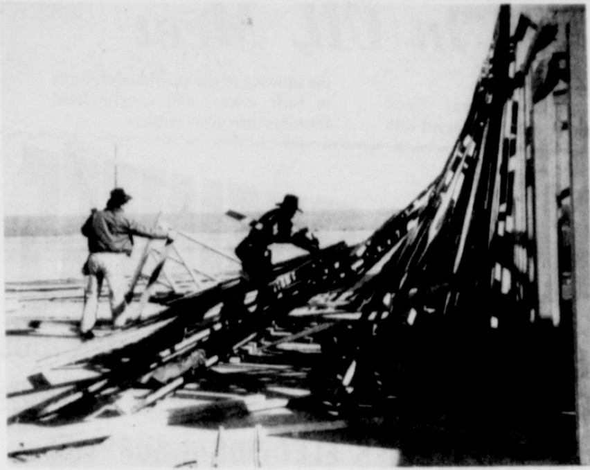
STORM DAMAGE.... The high wind of Monday toppled the framework for the garage at the new residence under construction by B.K. Buske on West 11th Street. Workmen are shown as they removed the damaged framework.
