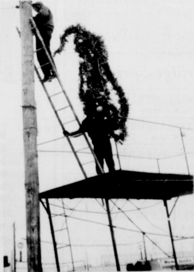
UP THEY GO....City of Friona employees braved the cold temperatures earlier this week, to put up the street decorations on Main Street. New pole decorations are being featured this year.
