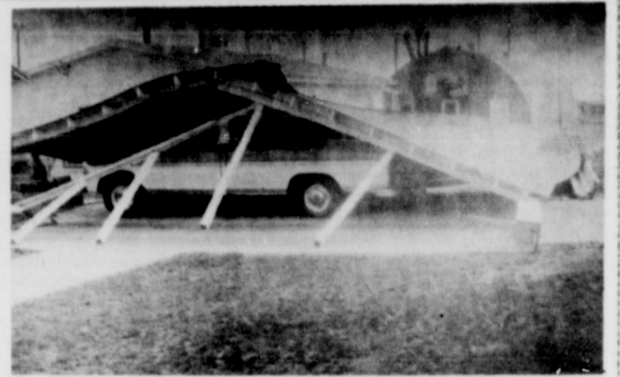
WIND DAMAGE...This carport, at the Gladys Wilson residence, collapsed during Tuesday's windstorm, trapping the pickup underneath. This was just one example of the damage done by Tuesday's wind.
