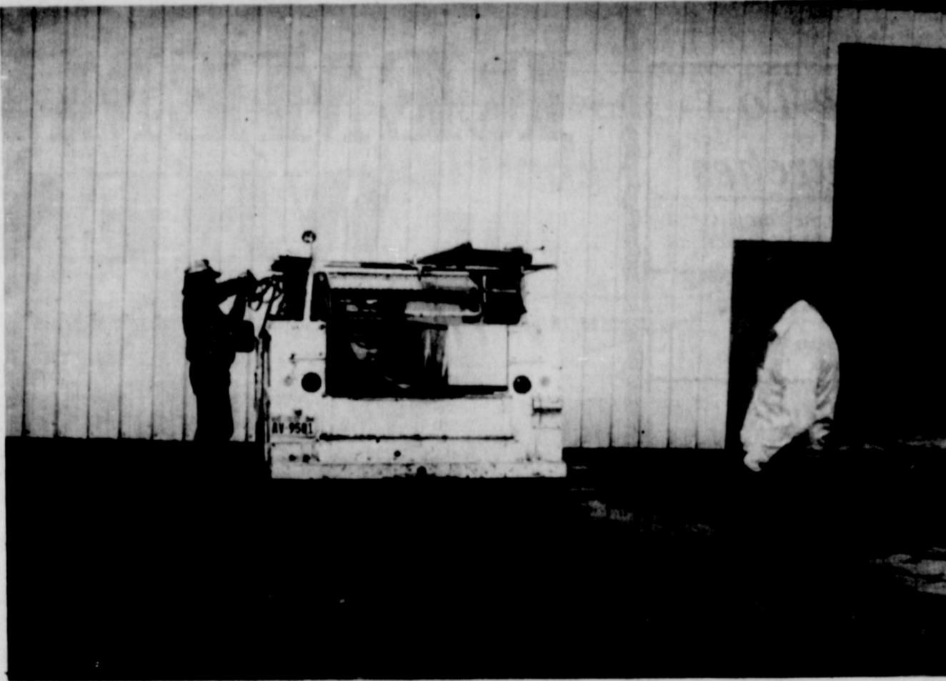
ADDITION GOES UP.... Roger Wilcox, owner of Friona Ford Sales, Inc., surveys the scene as a new shop building has been erected behind the company's present building.
