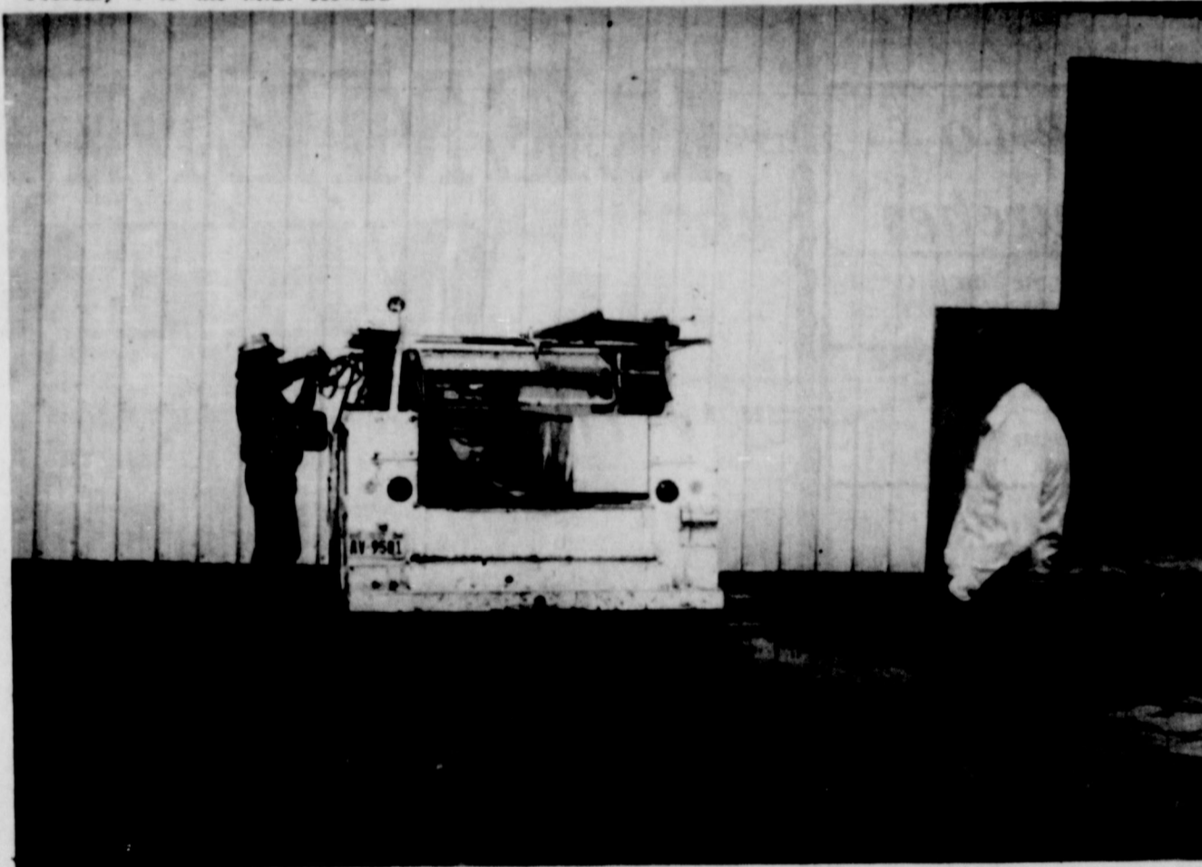
ADDITION GOES UP.... Roger Wilcox, owner of Friona Ford Sales, Inc., surveys the scene as a new shop building has been erected behind the company's present building.
