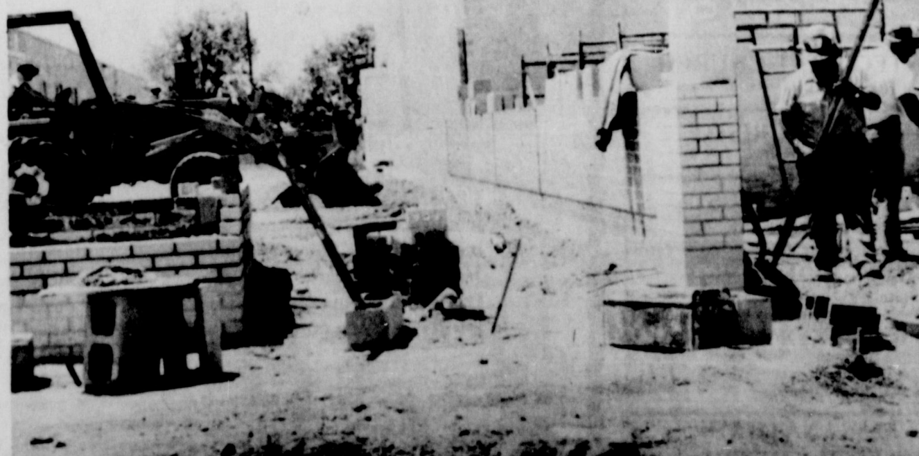
WORK UNDERWAY.... Construction is underway on the new school cafeteria for Friona Junior High and elementary school, and workmen have sand-blasted the adjacent auditorium-gymnasium to give the bricks a new appearance. Blessed by good weather the past few weeks, work has progressed well on the $1 million project.
