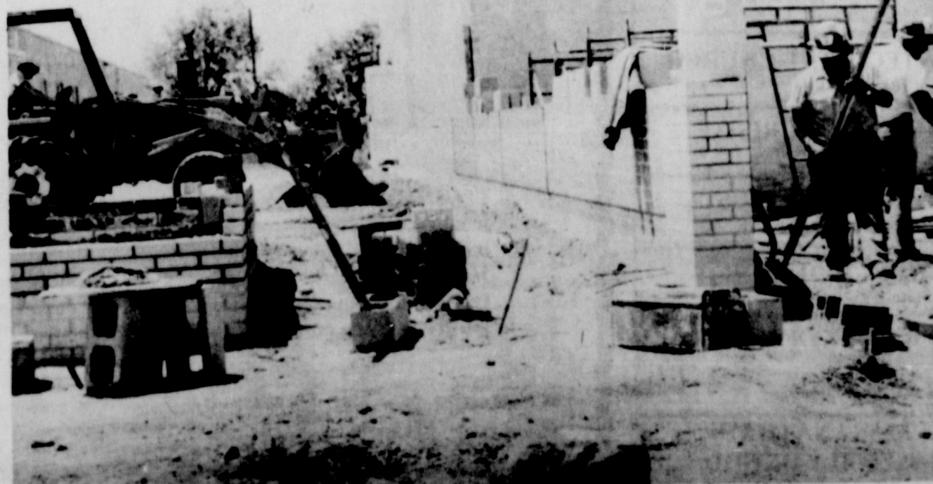
WORK UNDERWAY.... Construction is underway on the new school cafeteria for Friona Junior High and elementary school, and workmen have sand-blasted the adjacent auditorium-gymnasium to give the bricks a new appearance. Blessed by good weather the past few weeks, work has progressed well on the $1 million project.
