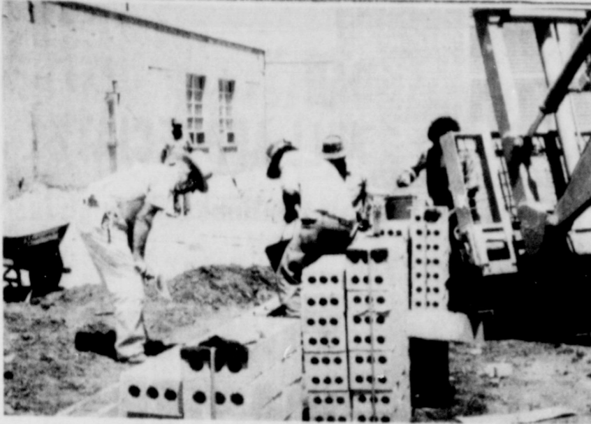
CONSTRUCTION... Workmen are shown laying bricks on part of the construction underway at Friona Junior High. The work is progressing nicely on the project, which will provide a new school lunchroom along with new classrooms. The buildings are also being renovated as part of the project.
