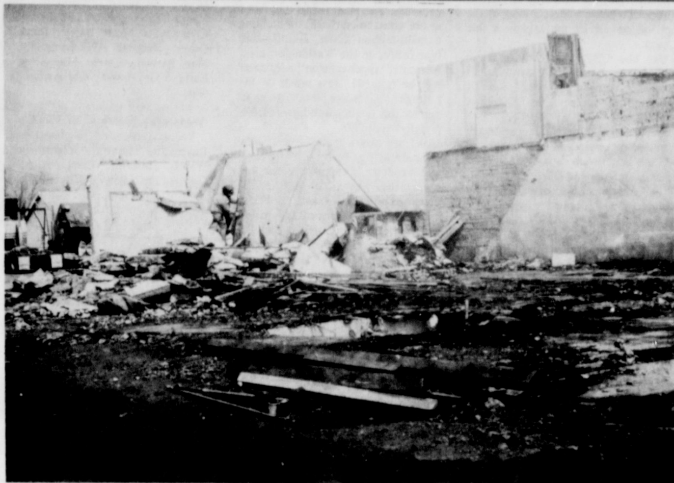
COMING DOWN.... The old building on U.S. Highway 60 at Washington Street was being torn down this week. For the last several years, the building has been mainly an "eyesore," and its razing will be a big improvement to the neighbors and the highway as seen by passers-by.
