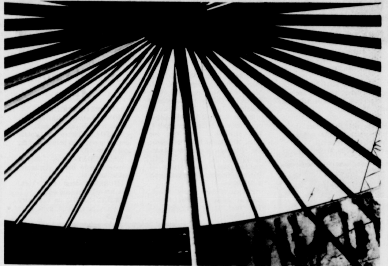
STEEL WEB...What appears at first glance to be a possible domed stadium for the Friona area is actually the new million-gallon water tank with the roof girders in place. Work on the giant tank continues to proceed. The bid was awarded on the pump station at a special meeting of the City Council this week.
