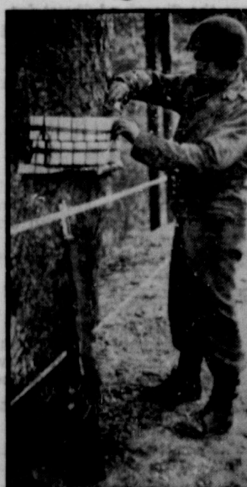
Pvt. John B. Brady of Philadelphia, Pa., and the 203th combat engineer battalion puts a charge around a tree in a defensive position near Bouissonville, Belgium. The explosives are placed in such a way that when set off the tree will fall across the road. (Signal Corps photo.)
