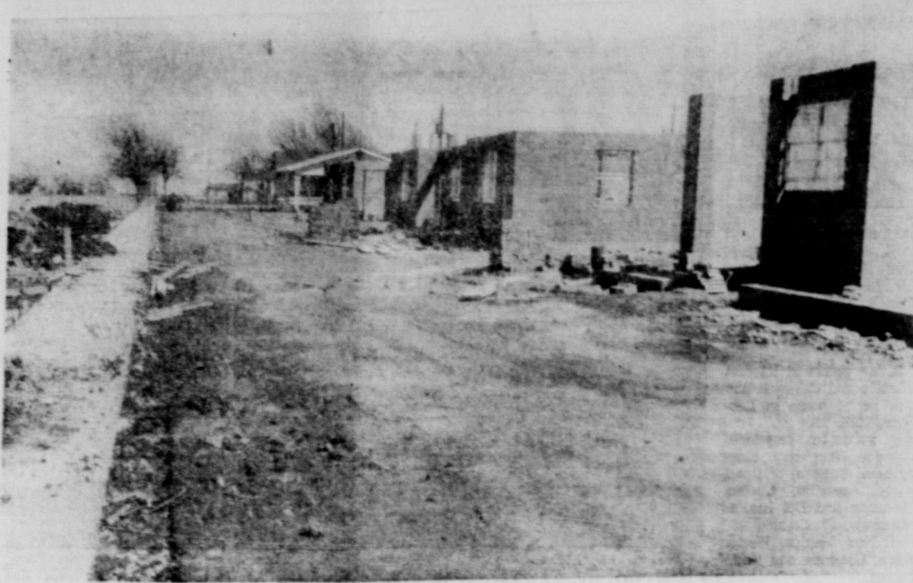
THE FLOYDADA LOW RENT HOUSING PROJECT is progressing about on schedule. When this shot was made a few days ago report from the builder was that the overall job was a little more than 50% completed. The picture shows buildings on east Tennessee Street. When the job is completed this summer it will represent an expenditure of more than $400,000 and will offer housing to a number of families.
