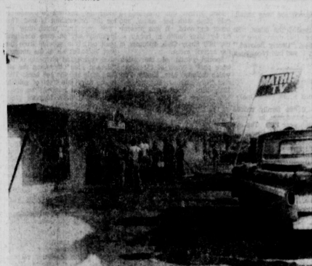
FIRE AT MATHIS TV ... Floydada firemen quickly extinguished this fire that developed Thursday afternoon. It was confined to extensive damage to the interior of the business.
