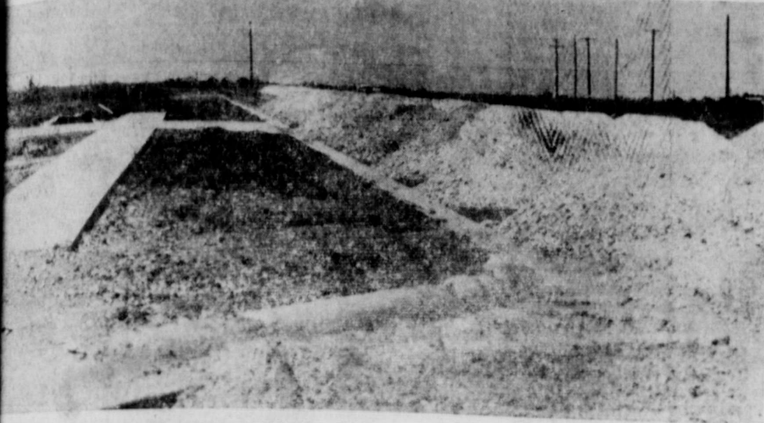
BUILDING ADDITION . . . Paving is almost complete on the new building addition in southwest Floydada of Wayne Williford, building contractor. Williford has started building one house at the west end of the street while paving is being completed.
