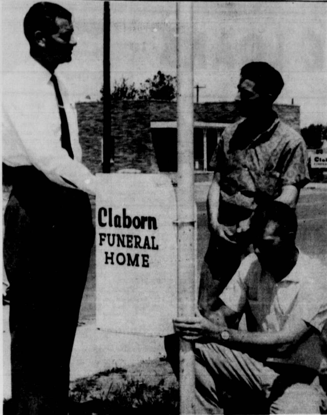
TRASH CATCHER!!! Jay Claborn was the sidewalk superintendent during erection of a Litter Maid trash receptacle on Main Street one day last week. Putting final screws in place is Bill Dufur, Litter Maid sales director. Vaughn Killian, field director is also pictured.
