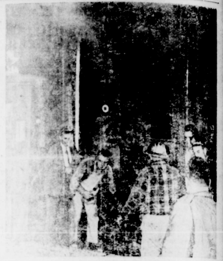
WORKERS RUN AWAY from a tunnel project in Boston after an elevator shaft fell 400 feet from the shaft and killed three men 400 feet from the surface. The men were not aware of their peril until the shaft plunged above them. They were brought out without injury.
