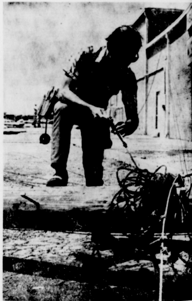
Telephone installer surveys damage to telephone in suburban Corpus Christi.
