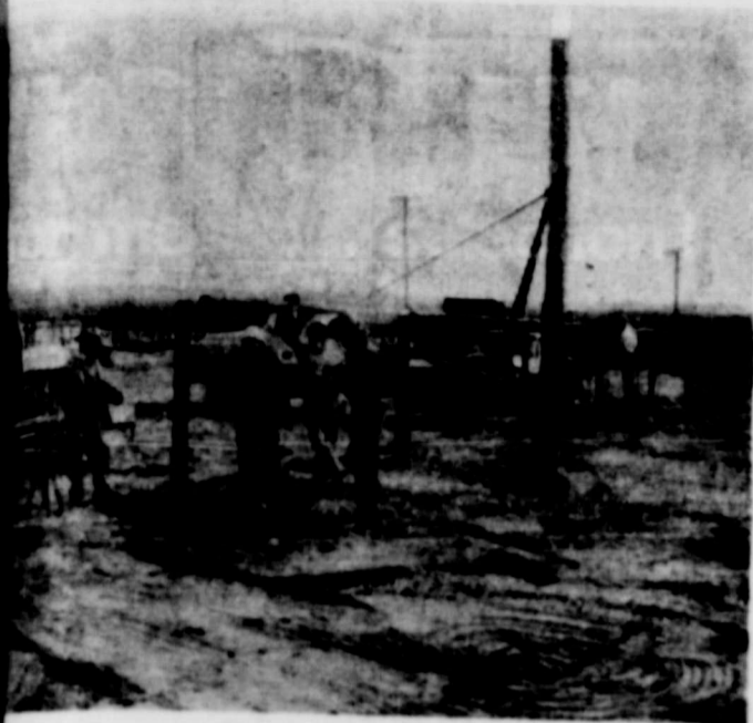
BUILDERS AT WORK —Volunteer workers are installing a pipe-frame fence at the Dub Day 4-H Rodeo Arena. Working Saturday on the job: Frank Absher, Billy Bearden, Eddie and Jake and Kirby Shipp.
