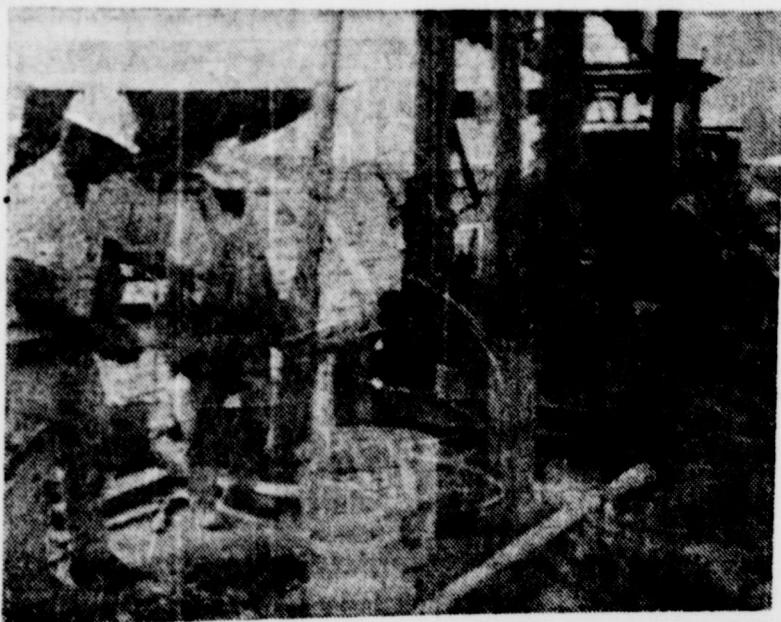
Pictured above are Sam Fitzhugh (l) and driller I. O. Fannin as they operate the bailer on a well being drilled on the Grover Yocham property just east of the Rankin Country Club.
