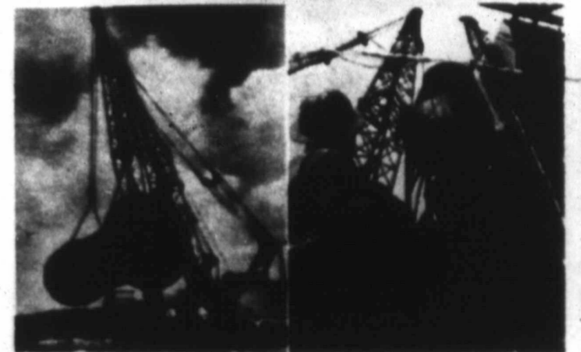
CHICAGO — The world's largest hot blast cupola is shown here being moved and set in position at Arme Steel Company's oxygen steelplant here. A cupola is a giant melting pot where scrap and other ingredients are melted into molten iron. The cupola has several sections; will stand seven stories high when completed, and will process 50 tons of molten iron an hour. The main section alone weighs 65 tons. Built by Drave Corporation of Pittsburgh, the big equipment is part of a $4 million facilities improvement program recently announced by Arme.
