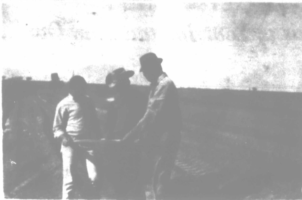
STUDYING LAYOUT of the parallel terrace system on the Bess Rorr farm is, from left to right, Mike Mudgett, SCS employee from Sudan; Roy Dolle, Littlefield farmer; David Thompson, Littlefield contractor.
