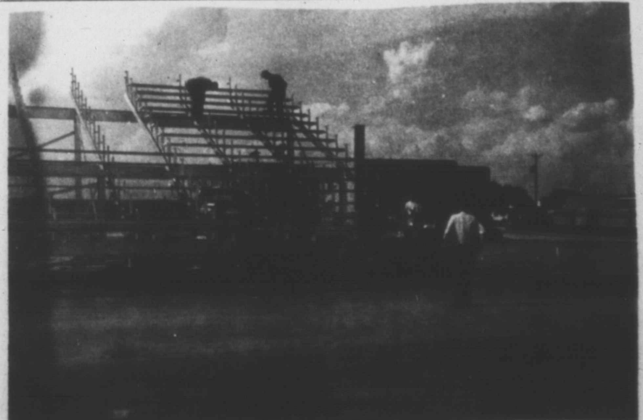
FOOTBALL STADIUM CONSTRUCTION -- New football stadium grandstands are nearing completion this week, as work continues on the Sudan School remodeling and building program.
