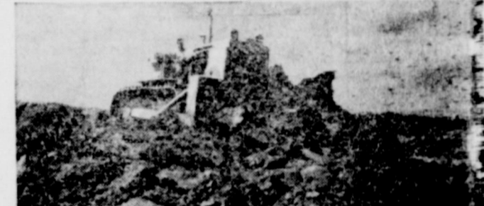
BEAR for work is this new International TD-20 crawler tractor here moving huge load of earth on runway extension project at Chicago's jet-age O'Hare International airport.
