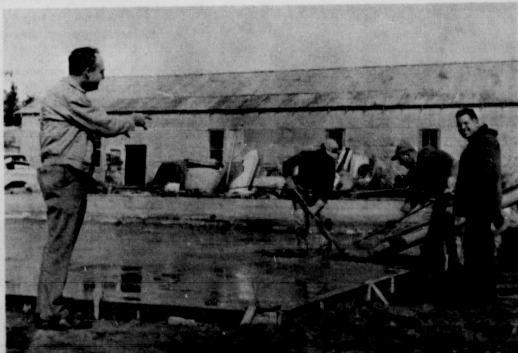
COFFEY BUILDING . . . Leonard Coffey (left) and Leon Coffey (right) watch as Lewellen Construction lays a foundation for a new 40 X 90 steel building which the Coffeys are building just south of their present City Body Shop location.
