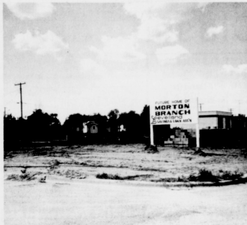
CONSTRUCTION GOT UNDERWAY this week on the new office building for the Morton branch of Levelland Savings and Loan located in the 300 block of south Main. The one story brick and stone building will contain 4,300 square feet of floor space which will house the necessary company offices and a 25'X57' community room. The community room will be connected to, but separate from the offices and will be open to clubs and organizations for their activities both day and night, company officials announced. Target date for opening is some time in November.
