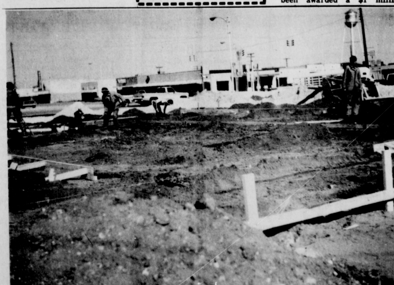
DON'T LOOK LIKE MUCH NOW, but it's what will come later that counts. This photo was taken as work got underway for the construction of A Dairy Queen restaurant at the corner of West Washington and South Main, where the former Byron Auto Parts and Jeters Hardware stores stood. No completion date has been announced, but judging from the first few days progress, it should be too long in the future.
