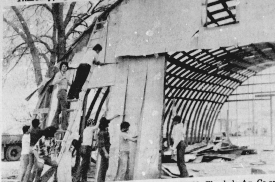
OLD COUNTY MAINTENANCE BARN COMES DOWN...Floydada Ag. Co-op Class of James Cleveland are pictured tearing down the old county maintenance barn to salvage material for their class projects. The remainder of the building barn to salvage material for their class projects. The remainder of the building came down on its own with the help of a high gust of wind Sunday. The crew is now busy taking out nails and hauling the material to the rodeo grounds to build smaller barns for chapter pens. Pictured are Rene Cruz, Donnie Morris, Mark Gilly, Terry Mayo, Tracy Turner, Blain Johnson, Rex Breed, Bud Taylor and Quinn DuBois.
