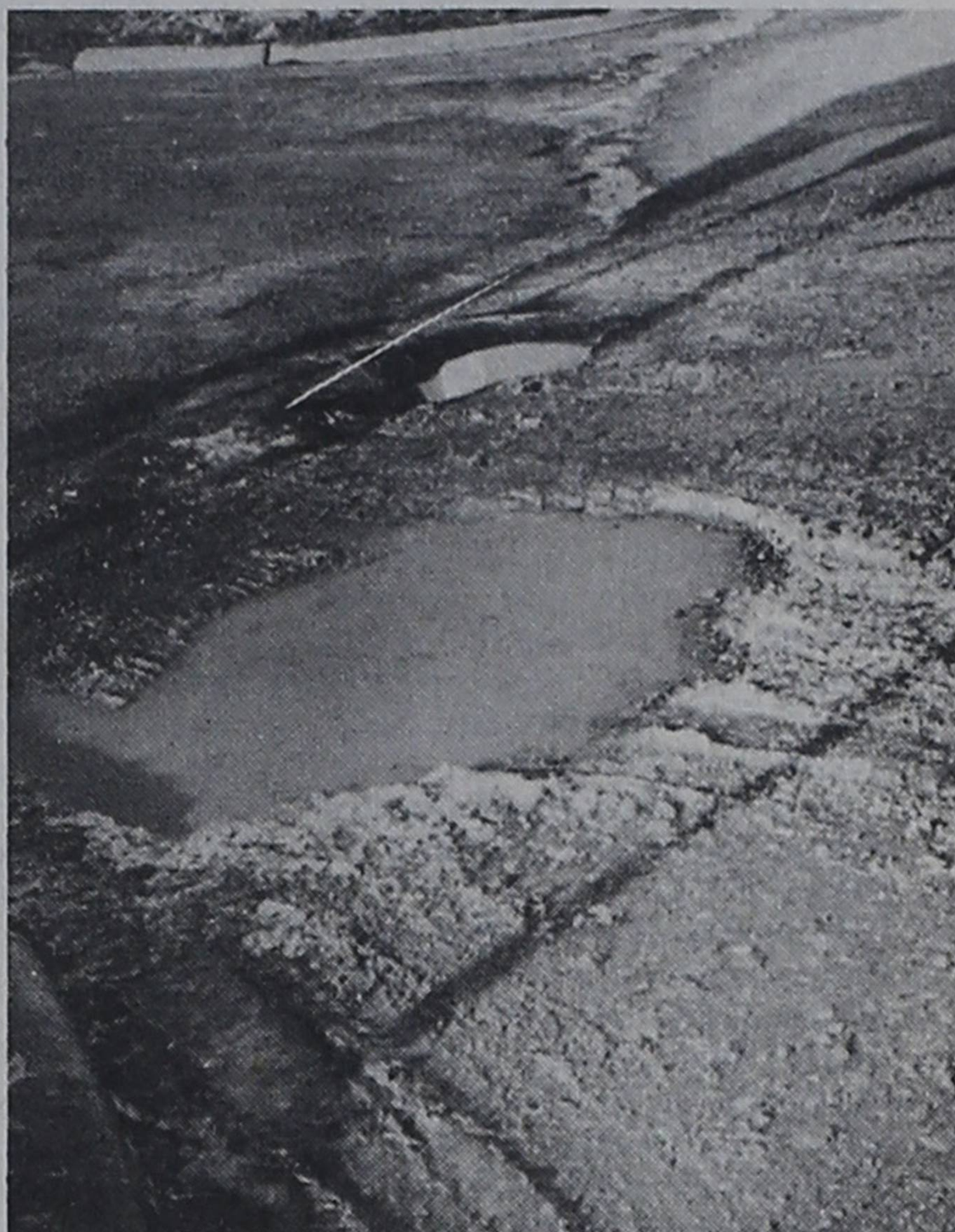
roof. The photo at the right shows one of many pot-holes which the city's streets and intersections have acquired. Parking lots also have been affected, and dirt roads in the area have been a big problem due to the snow.
