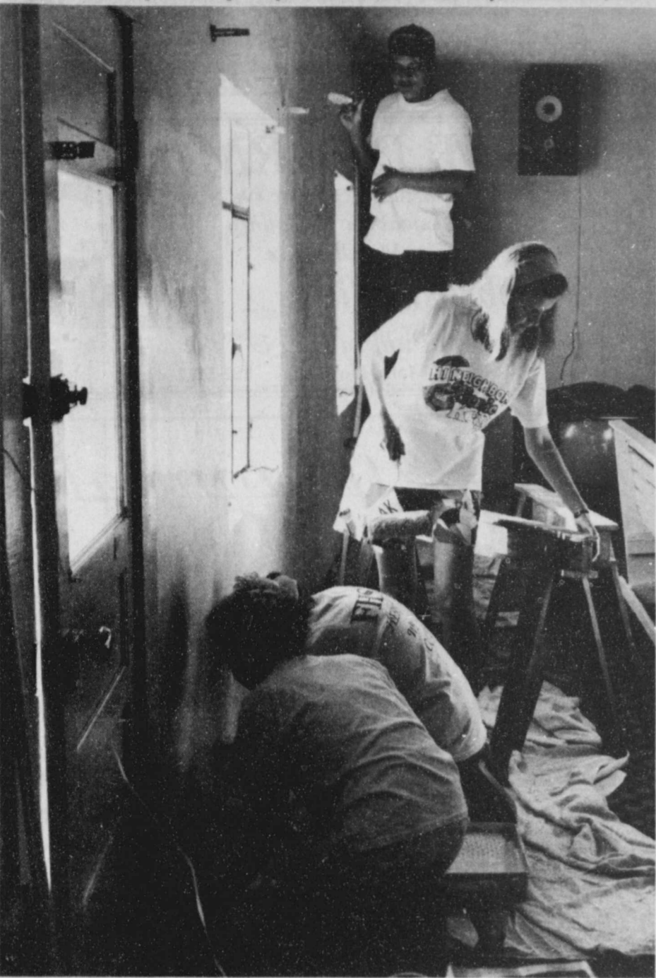
LENDING A HAND-- Members of the Floydada High School Student Council gave up part of their Saturday last weekend in order to help out the Floydada Senior Citizens with their building renovations. Students helping with the painting inside the building included (top to bottom) Chris Enriquez, Kjersti Tvinneheim and Laci Christian. Tvinneheim is this year's Foreign Exchange Student from Norway. --Courtesy photo
