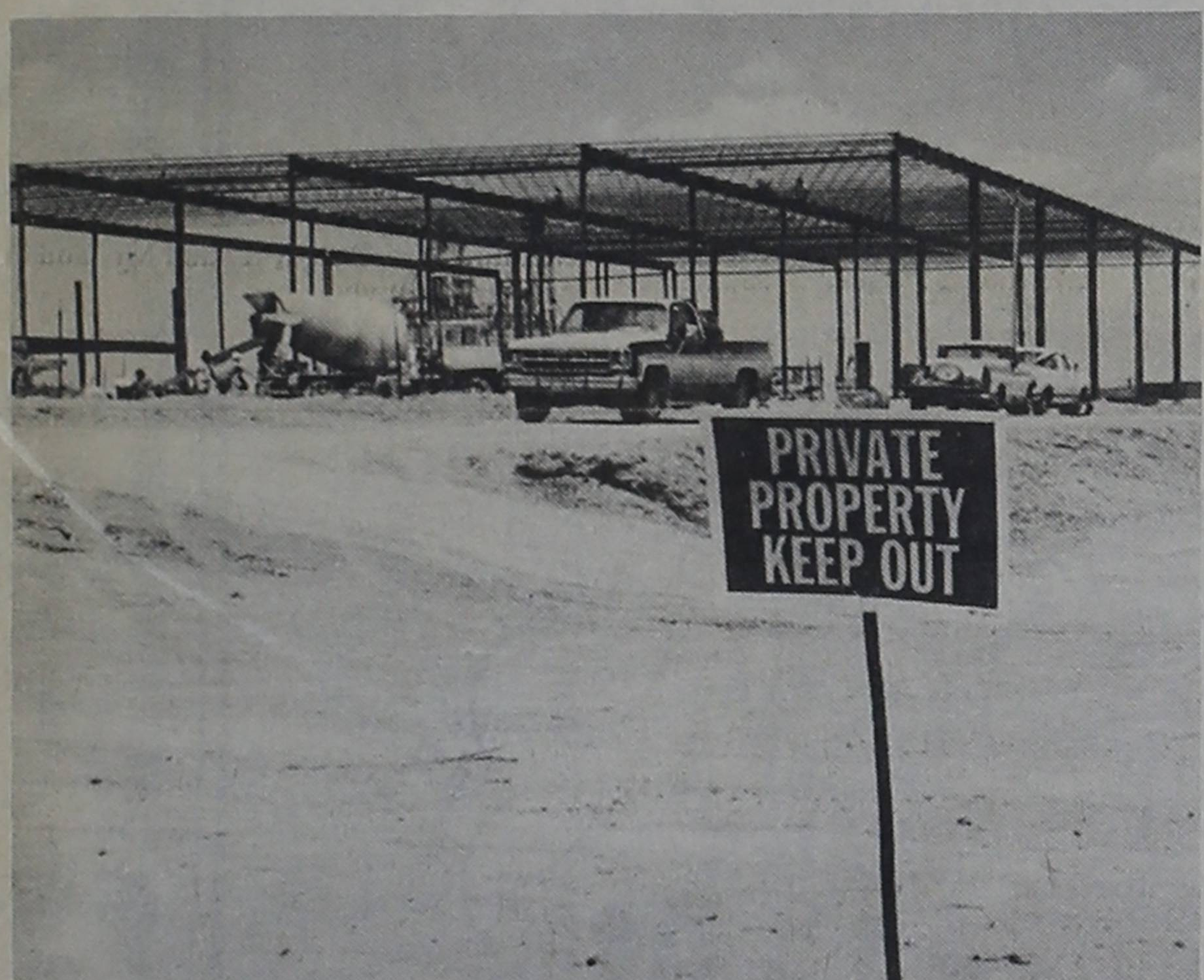
STEEL WORK BEGINS....Erection of the steel at the Millard Warehouse Complex was well underway this week. Meanwhile, a fenced strip with posted signs emerged during the past week adjacent to the western edge of the complex.
