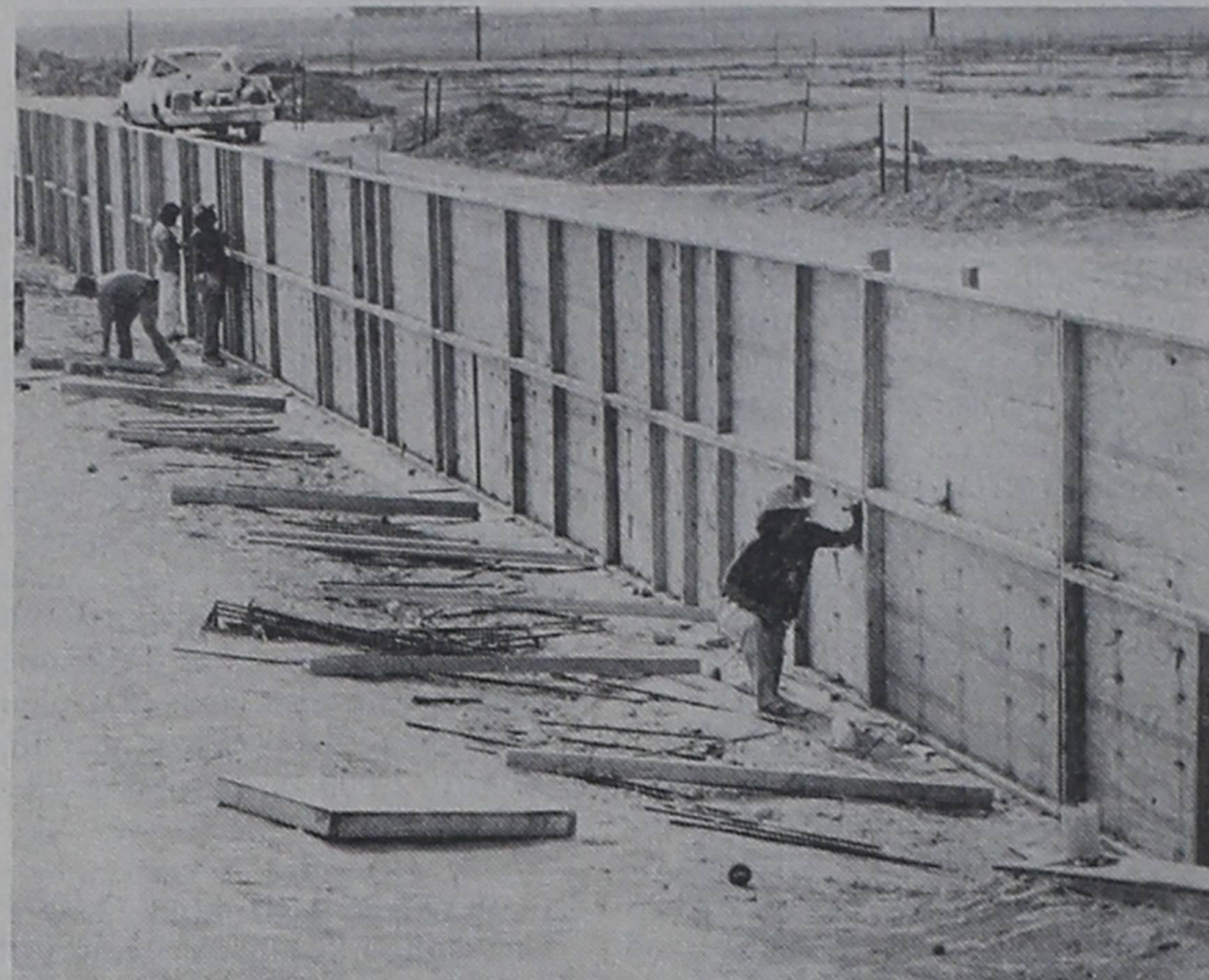
WORK CONTINUES... The foundation work at the new Millard Complex has made a lot of progress during the past week, as the new facility begins to take shape. Concrete forms are shown at the right, as workmen are busy in the foreground.
