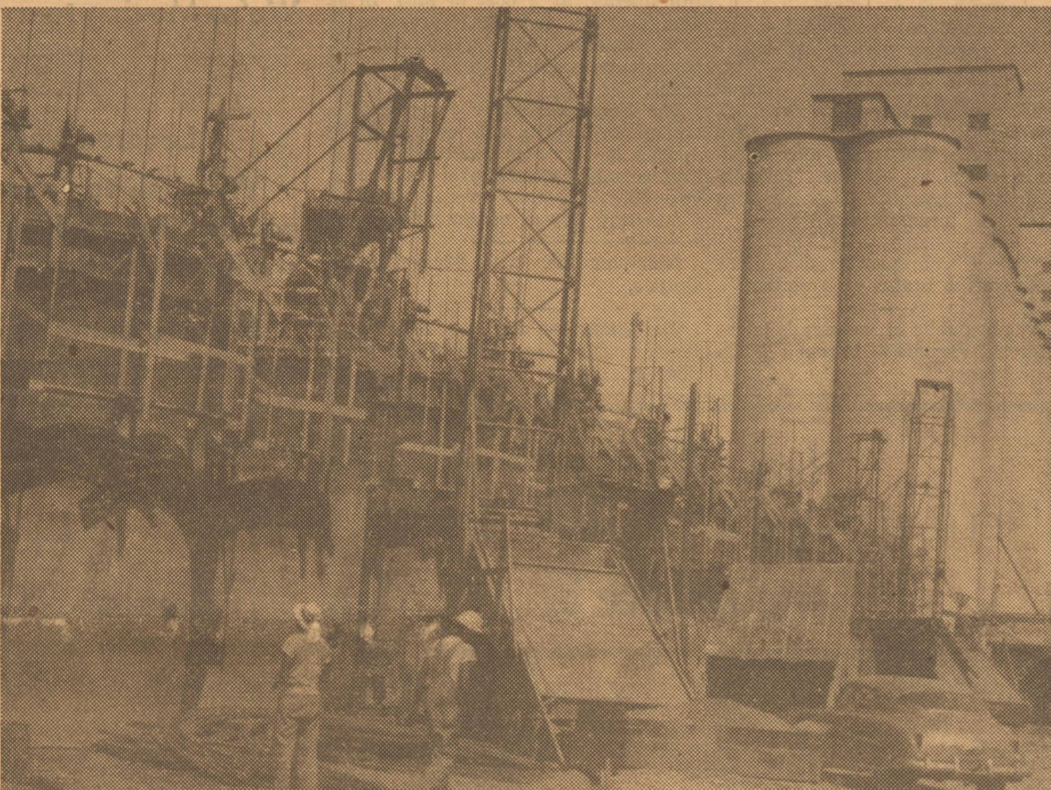
RIISING FAST —The concrete bins which will give Friona Wheat Growers another 1,000,000 bushels of storage are rising fast. Automatic hydraulic jacks "slip" the forms ever higher as fresh cement and reinforcing steel are joined.
