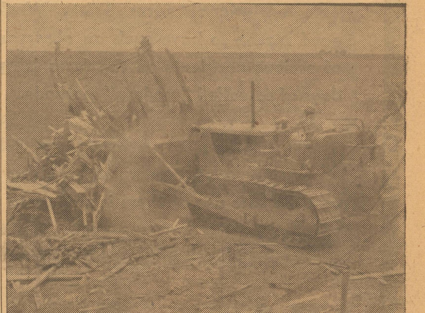
CONSTRUCTION STARTED—Removal of debris in preparation for relocating a dike along Frio Draw marked the first part of a million-bushel expansion of Friona Wheat Growers elevator this week. The bulldozer is clearing away form lumber left over from last year's expansion.
