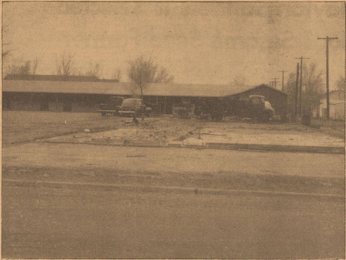
NEW MOTEL UNITS —This is the new east wing of Smiley’s Courts on Highway 60 in Friona. Most of the addition is up and workmen are starting on the inside details. The concrete in the foreground was a floor in the old Friona Motor Company building. Much of it will be used to serve as foundation for a new cafe in this location. Smiley Fulks says he plans to go ahead immediately with construction of the cafe.
