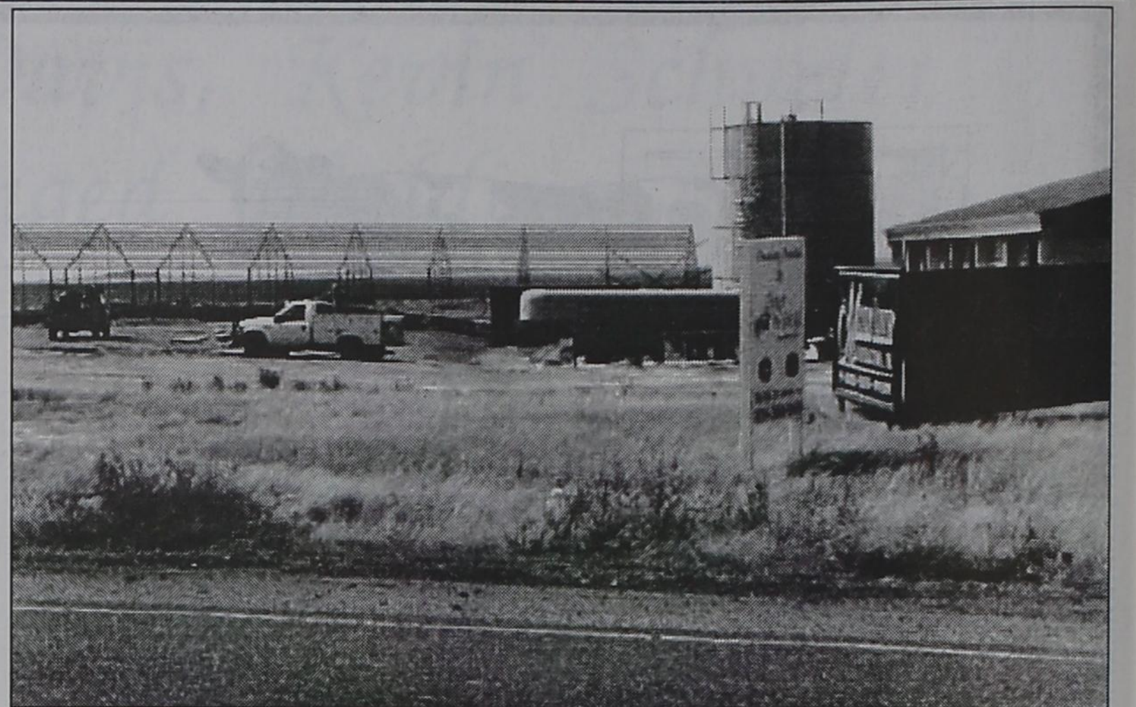
CONSTRUCTION is progressing on the High Plains Dairy located about 6 miles east of Hub on Highway 86. These views are taken looking south from the highway.
