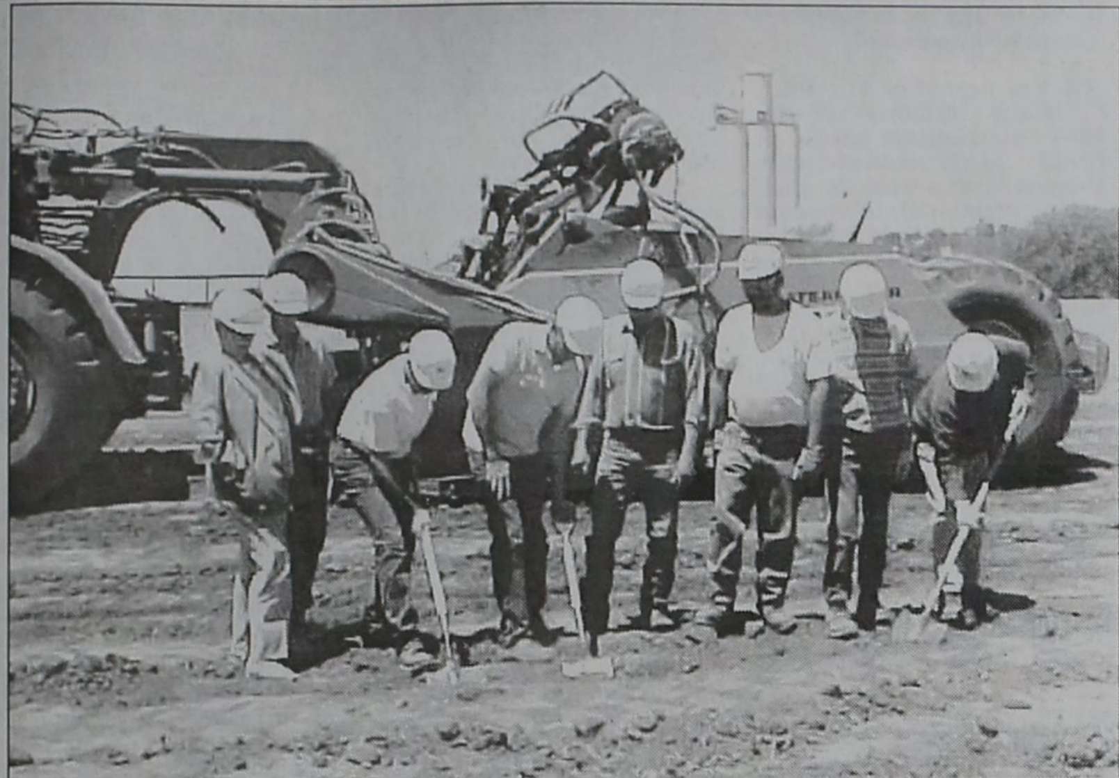
WEST FRIONA GRAIN employees gathered for the official groundbreaking of the new shuttle train grain elevator operation southwest of Friona. From left are Roger Denton, Freda Long, Terry Sharrock, Ken Rude, Jose Gonzalez, Rick DeLaPaz, Joseph Carpenter, Oscar Hernandez. See story for details. ron carr photo
