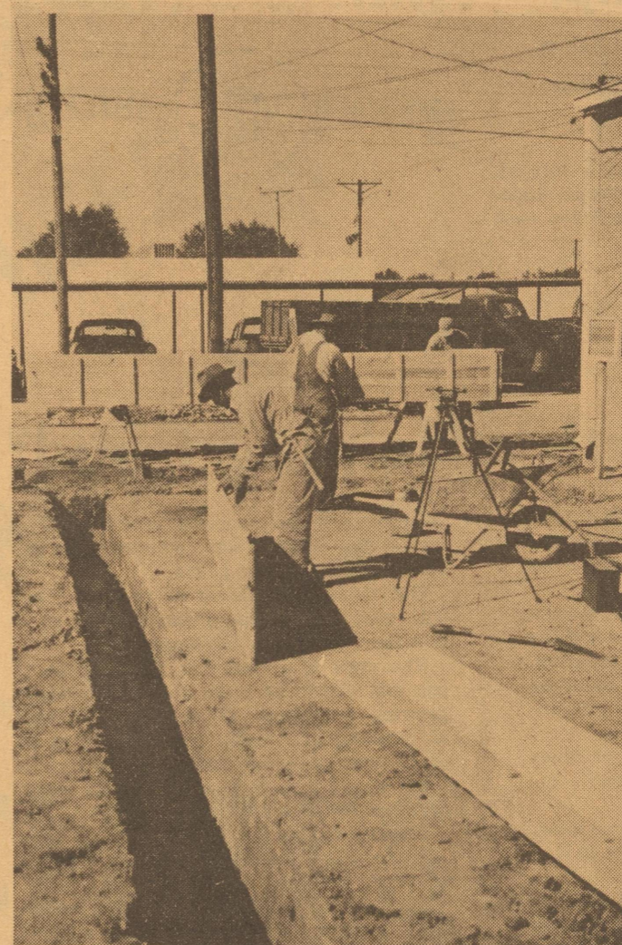
FRIONA STATE BANK'S ADDITION —Work got underway this week for the addition of a 50 x 18 room on the rear of the Friona State Bank that is designed for a community room. In addition the rear of the present building will be remodeled for drive-in banking facilities and a night depository.
