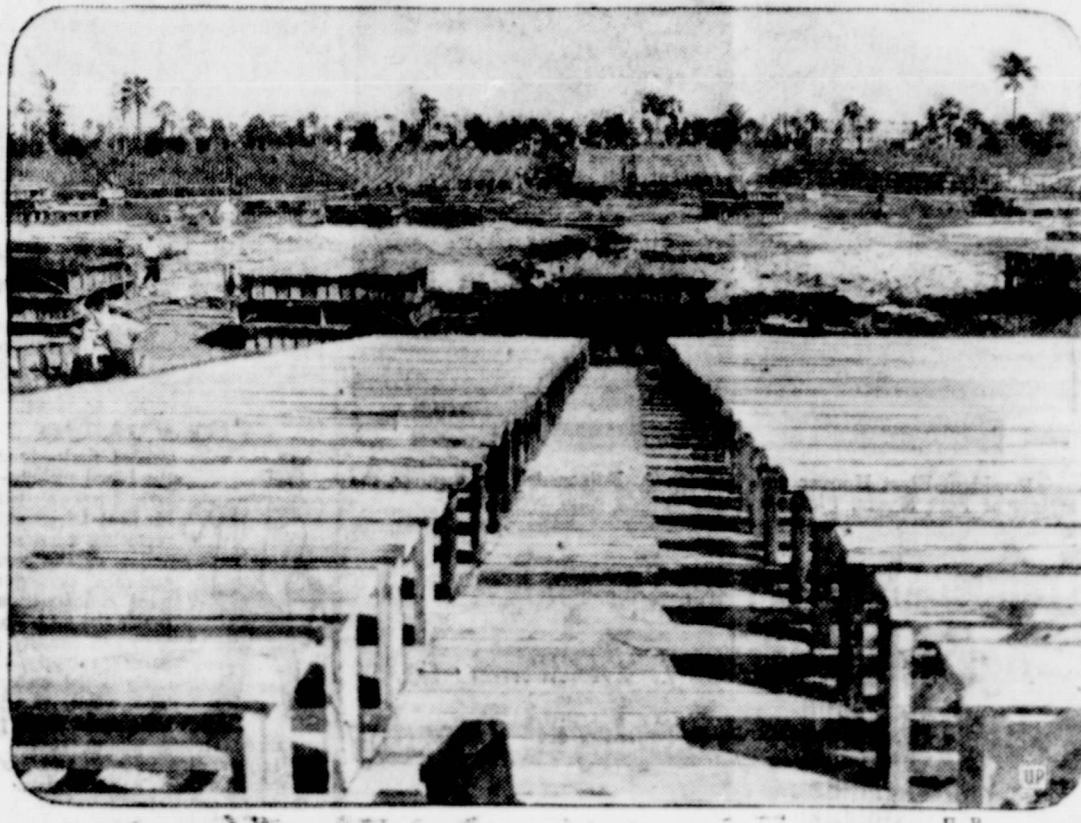
A view of carpenters and their assistants busily at work on the huge arena in Flamingo Park in Miami, in an effort to have it ready in time for the forthcoming bout between Jack Sharkey and Young Stribling on Feb. 27.
