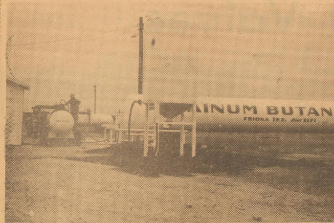
NEW SKYLINE LOOK --With the installation of a new tank to take care of Bainum Butane's phosphoric acid fertilizer the triangle west of town begins to take on a new look. Bainum installed the new tank this week.
